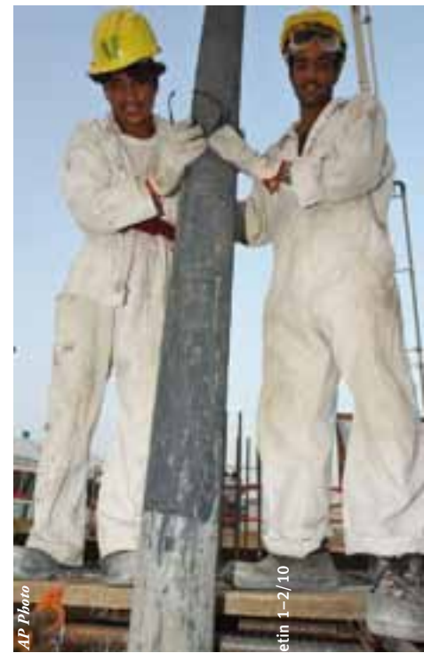
Construction workers hold the pipe during the first cement pouring ceremony at the foundation of the tower in September 2004.
